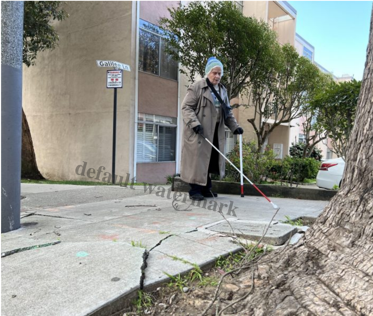
Gorman making her way around broken sidewalks on Laguna Street, near where she lives.
